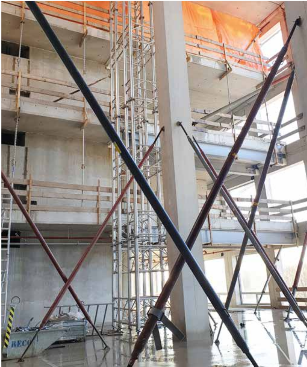
Precast concrete elements aligned and supported with TITAN RSK push-pull props (size 8 shown here) up to a height of 7.60 m
