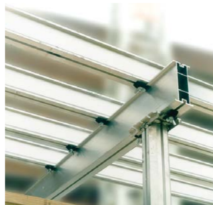
9. Position secondary beams and fix with a TITAN clamp at each intersection with a primary beam. Structure is now ready for fixing of plywood
