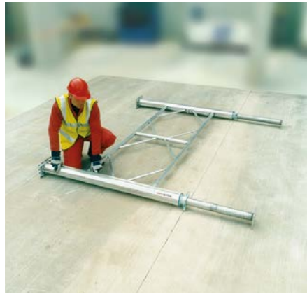
1. Connect ledger frame horizontally between two legs. Predetermined ledger frame position measured from headplate
